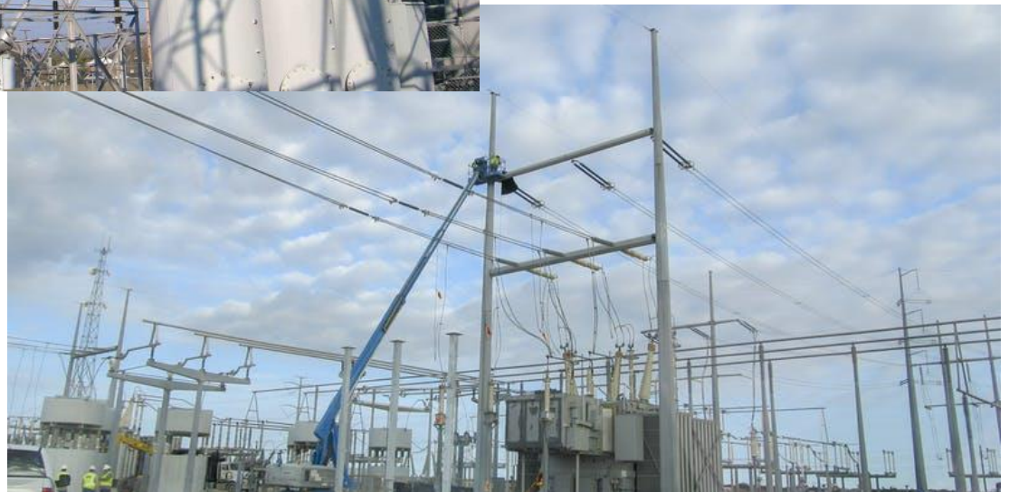
138 kV Substation OCB Rehab Waller, Texas >
