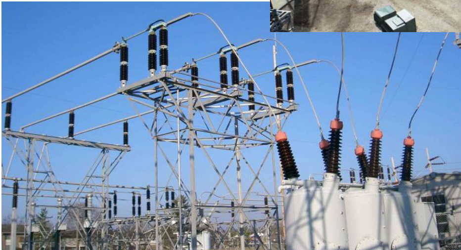
138 kV North Substation < Indianapolis, Indiana
