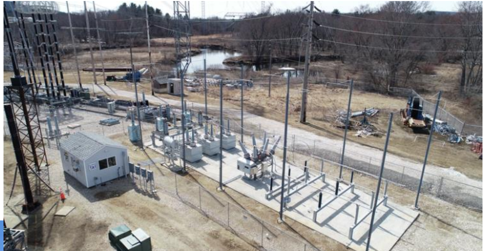
138 kV Research Substation Lenox, Massachusetts >
