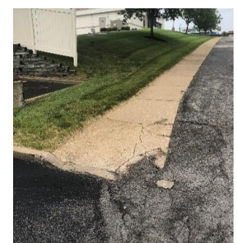
_____ Broken curb ramp (e.g. uneven walking surface)
