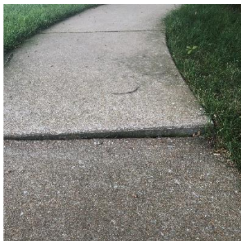
_____ Trip Hazards (e.g. uneven sidewalk panels)
