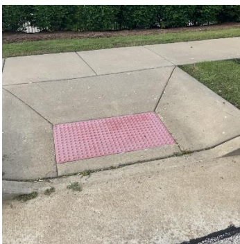
_____ Curb Ramp Grades (e.g. steep slopes)
