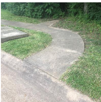
_____ No Curb Ramps (e.g. 6 inch drop off the sidewalk)
