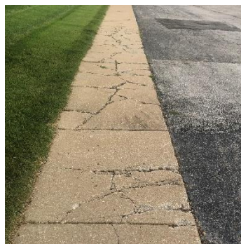
_____ Poor Surface Quality (e.g. broken sidewalks)
